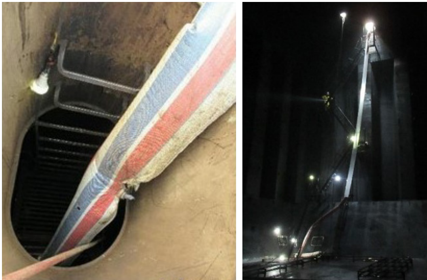
Figure 2: The entrance to No. 2 S COT (left) showing the vertical ladder inside the tank dome and the ventilation duct and cable. The access ladder inside the tank (right) showing the forward bulkhead, lighting and ventilation duct extending to the bottom of the tank. The pictures were taken on 22 May 2019. It was reported that the ventilation duct, cable, and lighting had not been moved since the ASD1's fall.
