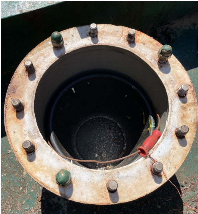
Figure 4: COT No. 5S Butterworth hatch with plastic bucket located inside and secured to threaded bolt with a wire.
