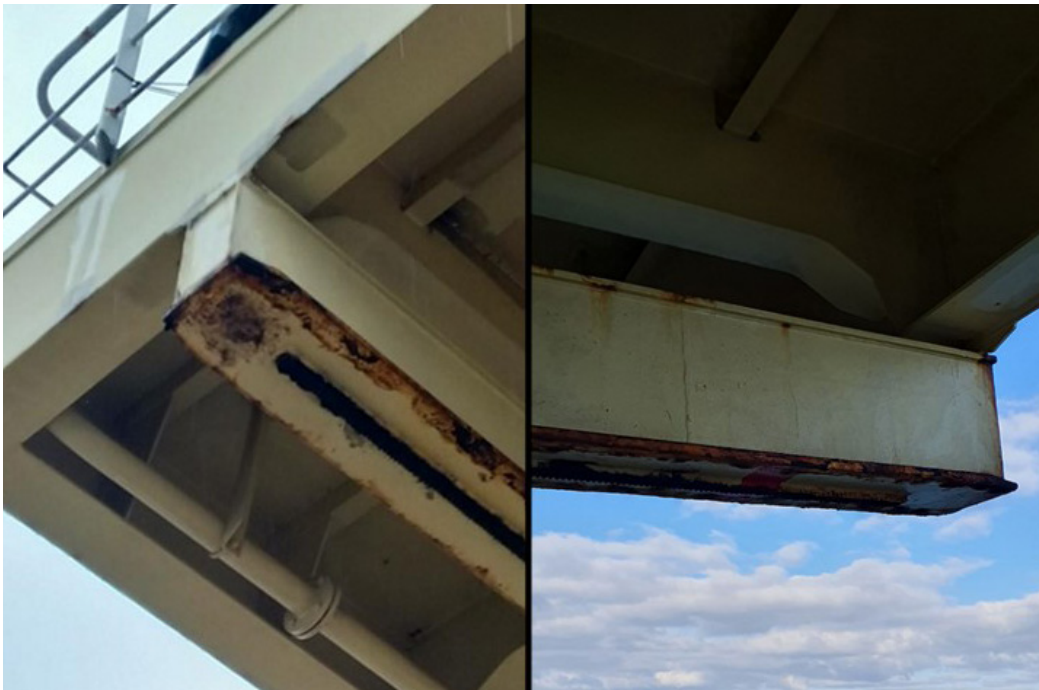
Figure 16: Photos of the forward side of the fixed monorail showing the lack of stoppers.
