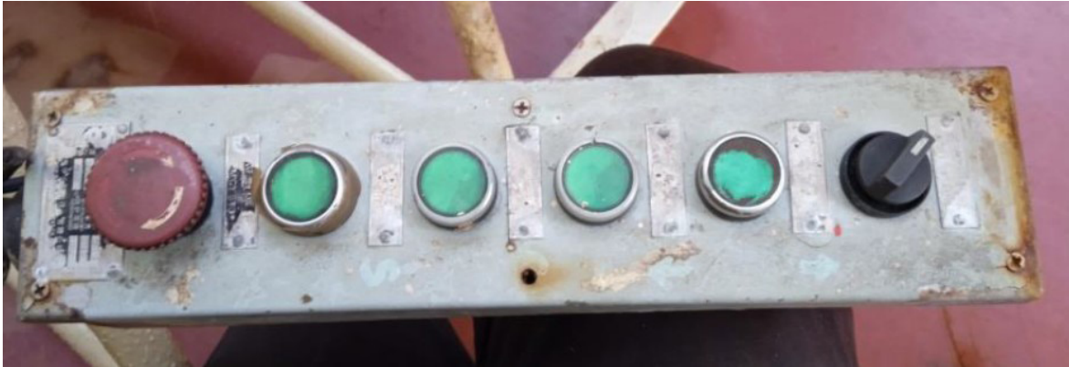
Figure 17: Controller for the provision crane.
