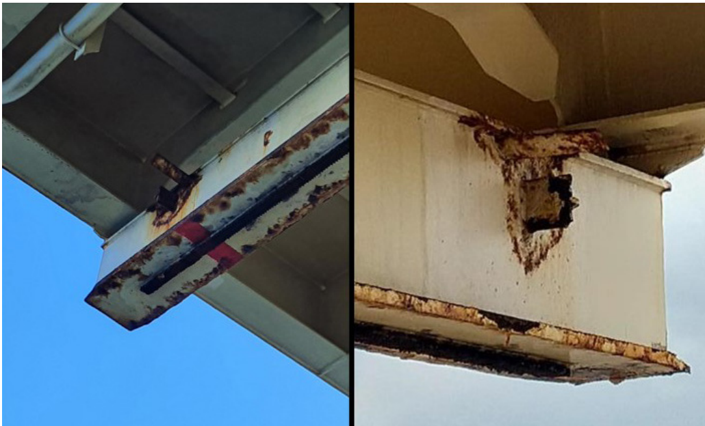
Figure 15: Photos of the aft side of the fixed monorail, showing the stoppers and the brackets to engage the limit switches.
