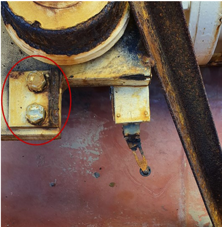
Figure 14: Photo of the limit switch on the aft, starboard side of the travelling gear assembly. The broken aft, starboard side stopper is circled in red.
