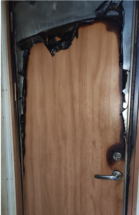
Figure 11: Photo of the inside of the door to the ASD1's cabin.
